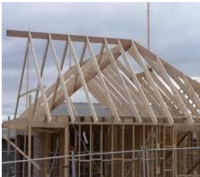
Figure 27: Conventionally framed with dimensional lumber, this roof has two gable ends, one valley and one hip. This roof will fare better than a lightweight roof during a fire.
