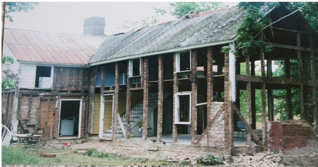
Figure 2: Balloon Framing: Studs extend from the foundation to the roof with minimal fire stopping.
