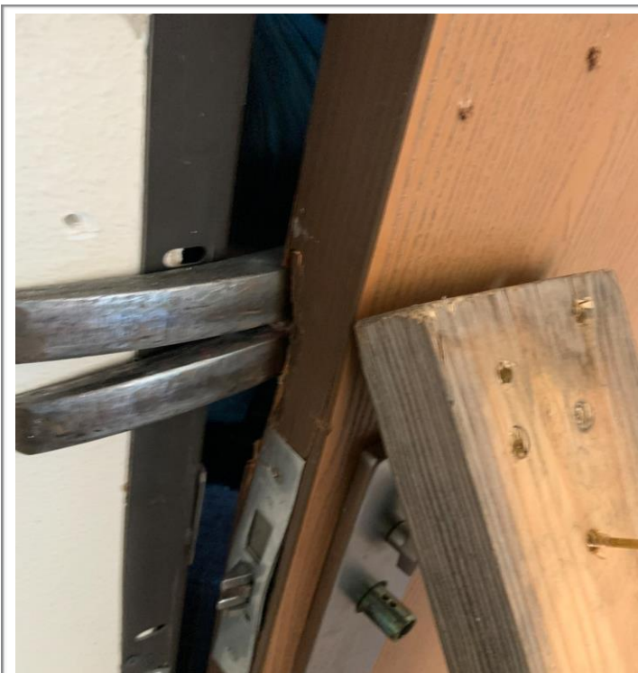
Excellent placement of the Forks in proximity to the locks, as well as, force placement.
