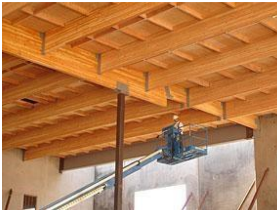
Figure 24: This is a typical panelized roof employing lam-beams for the main carriers, beams and smaller lam -beams for the purlins and 2x6 rafters.
