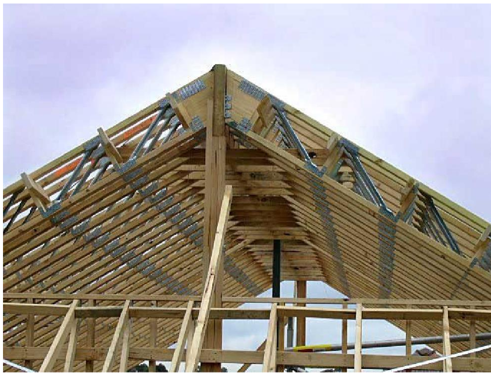
Figure 20: Parallel cord trusses come in many styles and are used in roof and floor assemblies.
