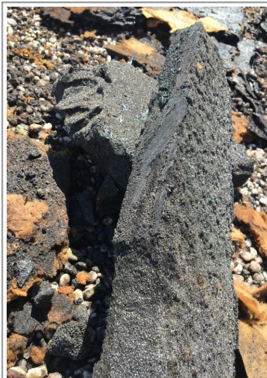
Fiberboard from a leaky roof that absorbed the asphalt membrane.
