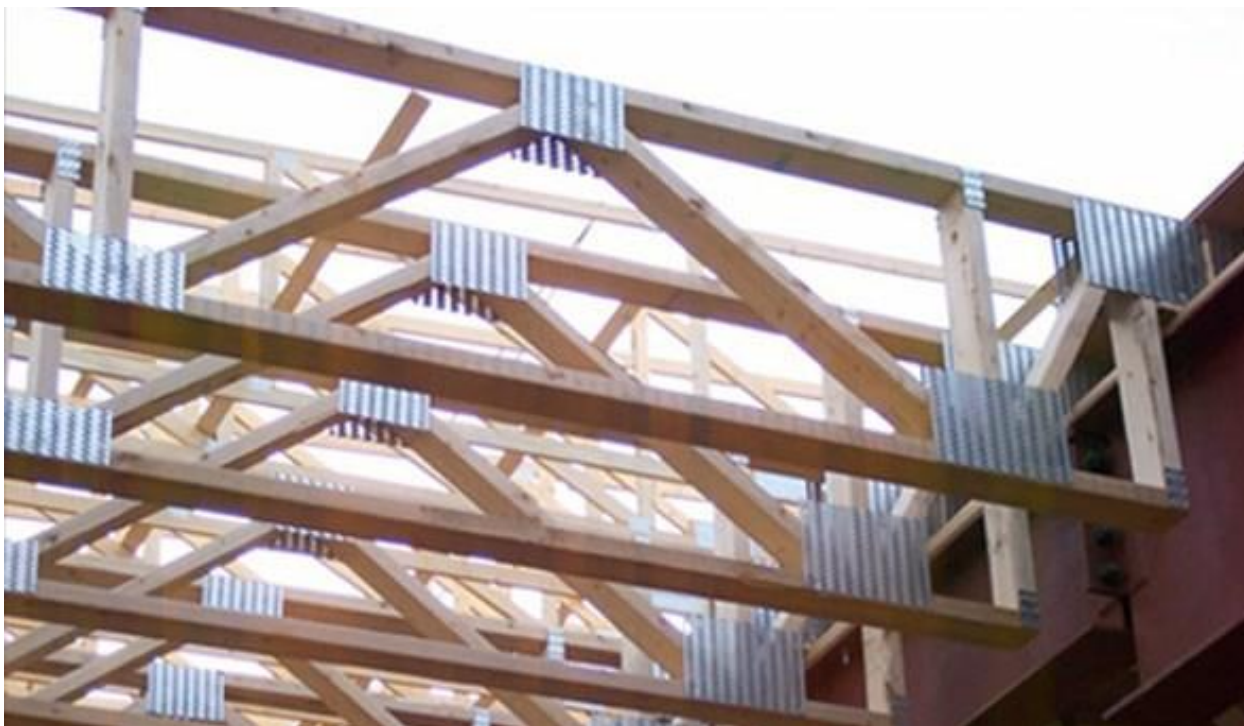
Figure 22: Open web wood trusses are often built with small dimension lumber and metal gang plates.
