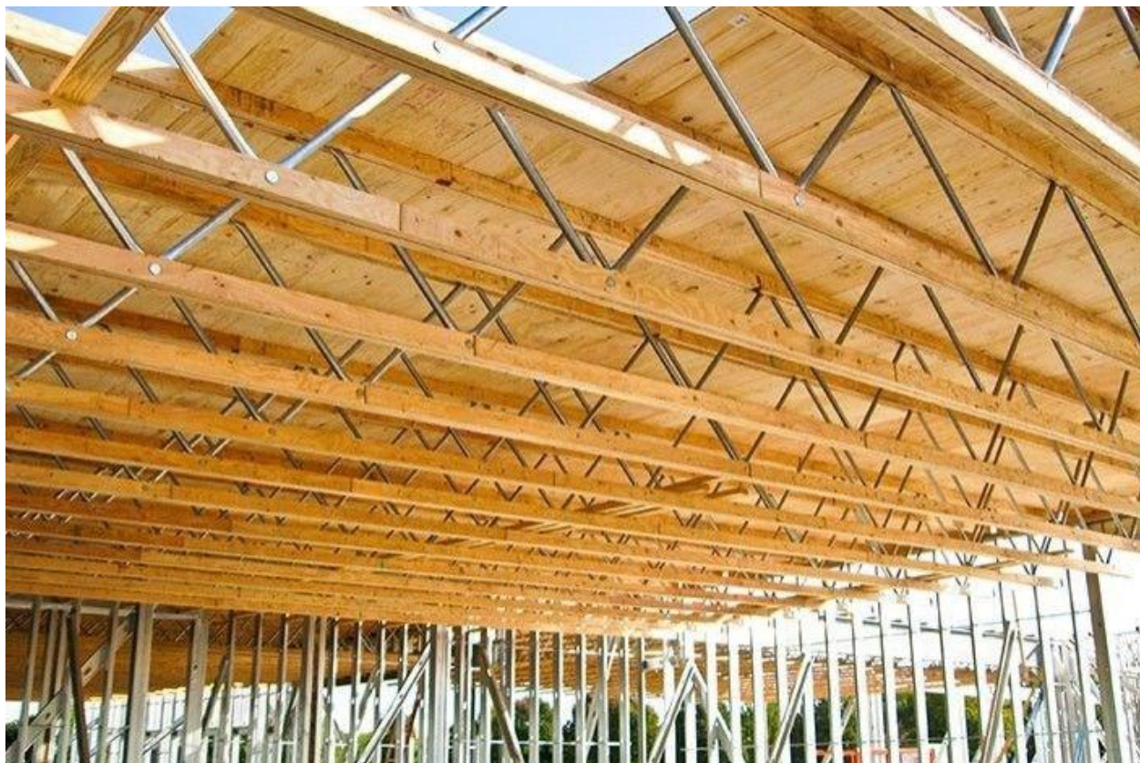
Figure 21: Open web metal trusses use lightweight metal to hold the top and bottom cords together.
