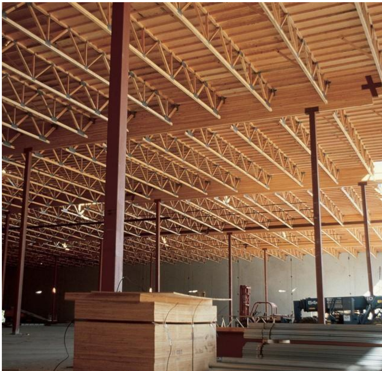
Figure 26: This hybrid system employs lam-beams for the main carriers and then lightweight open web wood trusses as purlins
