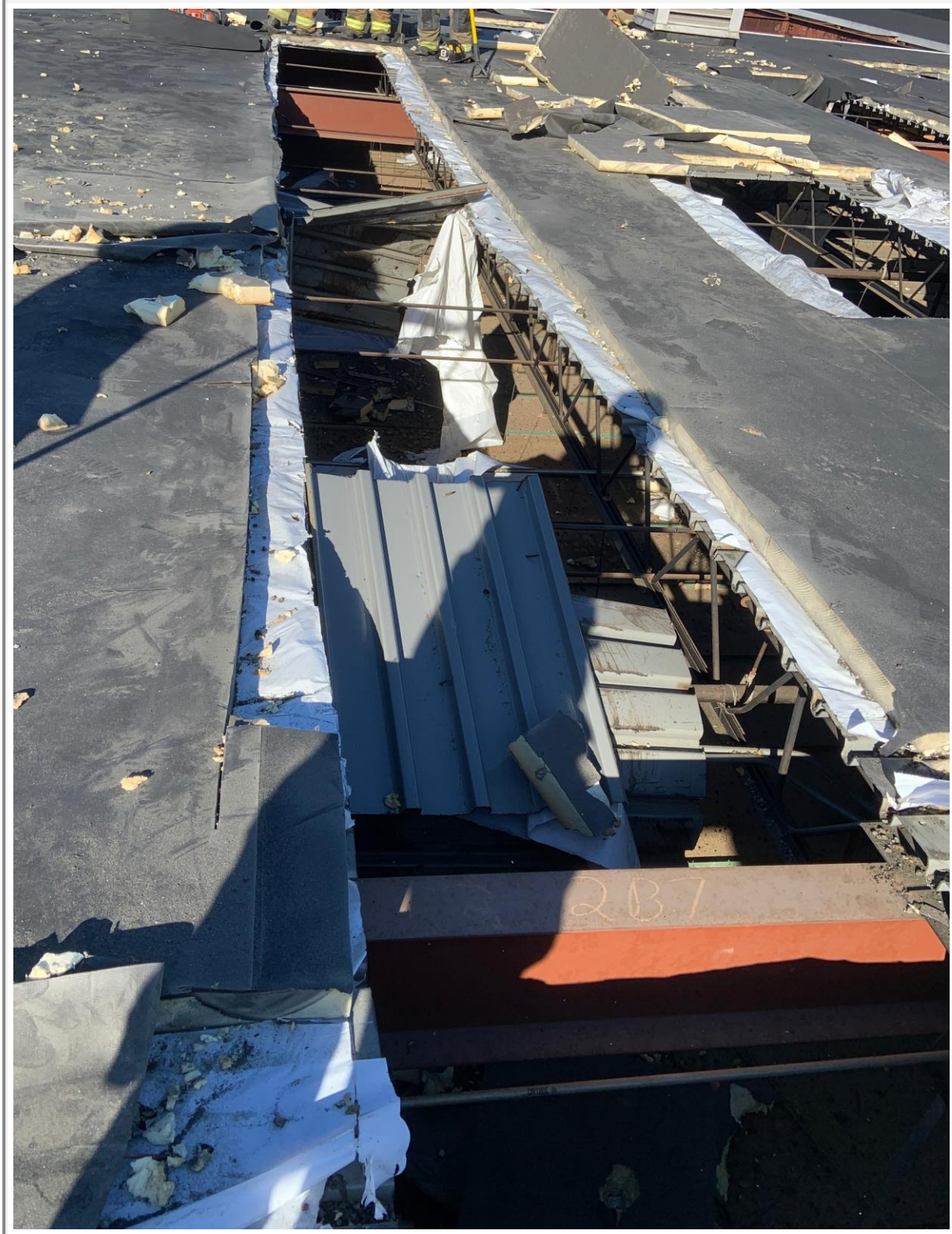
A 40 plus foot trench cut on a membrane based roof decking. This trench was a combination between a basic trench with construction and a “channel” cut.
