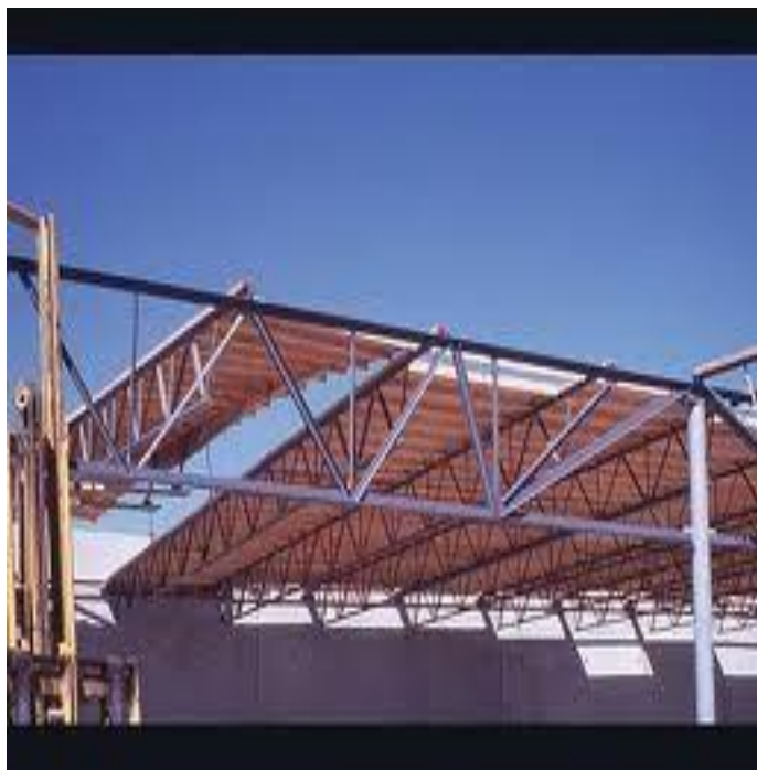
Figure 25: Lightweight panel system using steel bar-joist girder truss and steel bar-joist purlins.
